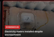
EVIDENCE #2 Electricity meters installed despite encroachment
